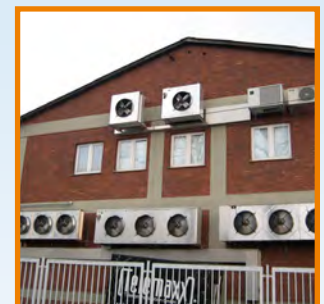
Multiple mounts of air conditioners for a computer center
